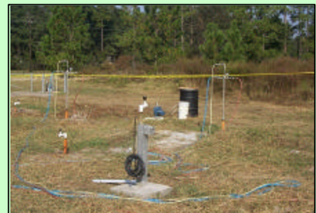
Figure 3: In-situ chemical oxidation injection wells (background) monitoring well (foreground).
