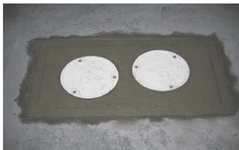
Flush mount injection well.
