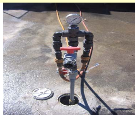
Standard GCI Injection Well Head
