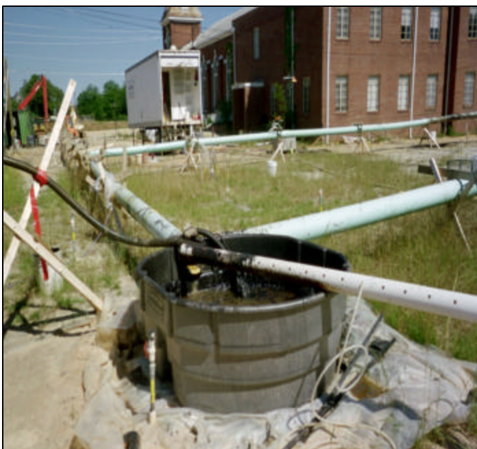
Water Collection System
